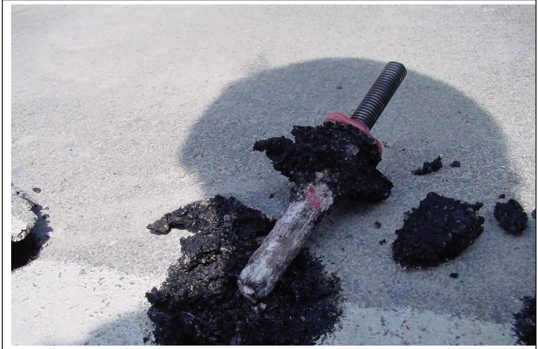
Fig. 3: A layer of asphalt approx. 1 to 2 mm thick is bonded to the HIT-RE 500 adhesive.
