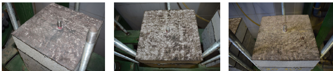
Figure 6. Surfaces of specimens no. 20.301 01 (left), 20.301 05 (middle), and 20.301 06 (right) after removing the ceramic tiles and the tile cement layers.
