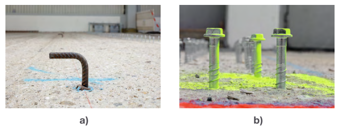
Fig. 7.12: Comparison between (a) post-installed rebars and (b) concrete screws used as shear connectors
