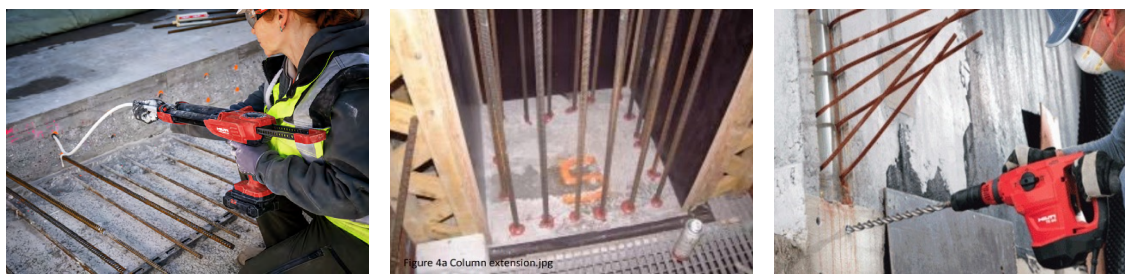
Fig. 2.3: Examples of extension of R.C. elements with lap splices using post-installed rebars
