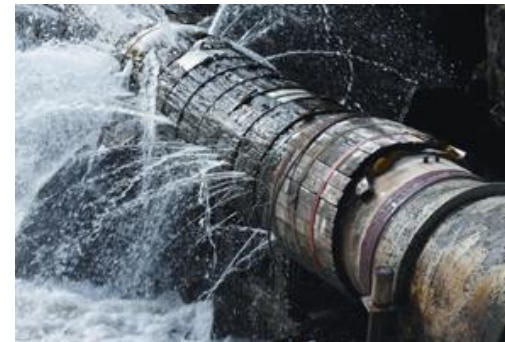
Mechanical forces (e.g. water hammer)
