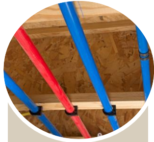
Water and Gas supply pipes
