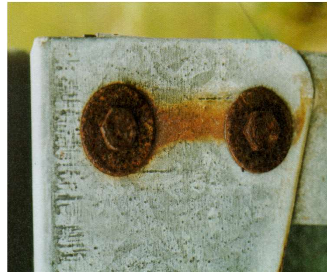
Hot-dip galvanised sheet metal (~ 30 microns) in coastal atmosphere and fastened with galvanised bolts (~ 7 microns)
