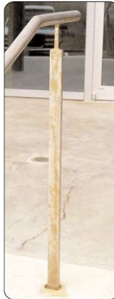
De-icing salt on parts near roads or in road tunnels
