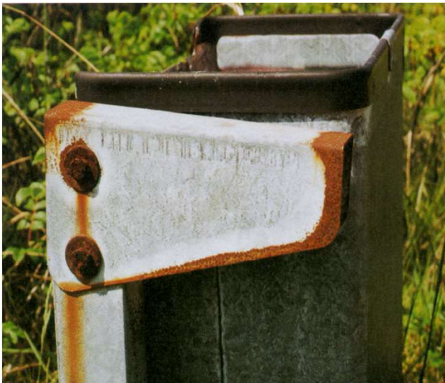
Hot-dip galvanised sheet metal (~ 30 microns) in coastal atmosphere - cut edges no longer covered
