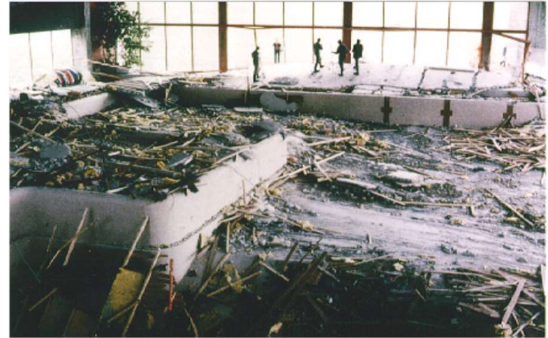
Collapse of swimming pool ceiling in Uster, Switzerland (1985) - Due to wrong design and material
