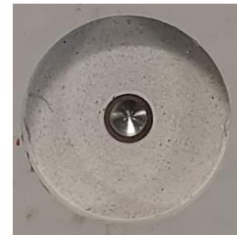
Locally exposed steel with shiny ring after PFP-removal operation
